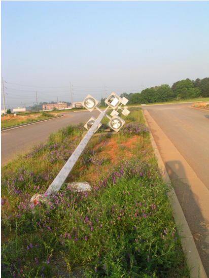
Light poles 30 feet tall await installation by electricians from Wayne J. Griffin Electric Inc. at Floyd College near Cartersville.
